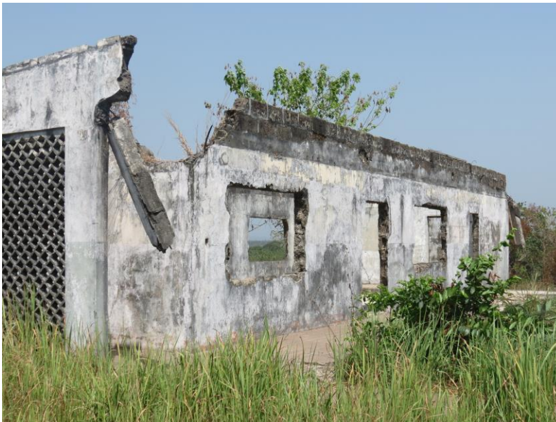
One of the Dilapidated Buildings in Teko
